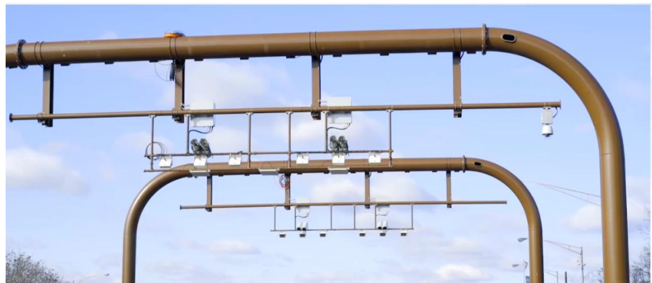
Figure 1-1: Example of Cashless Tolling Gantry Over a Mainline Roadway
